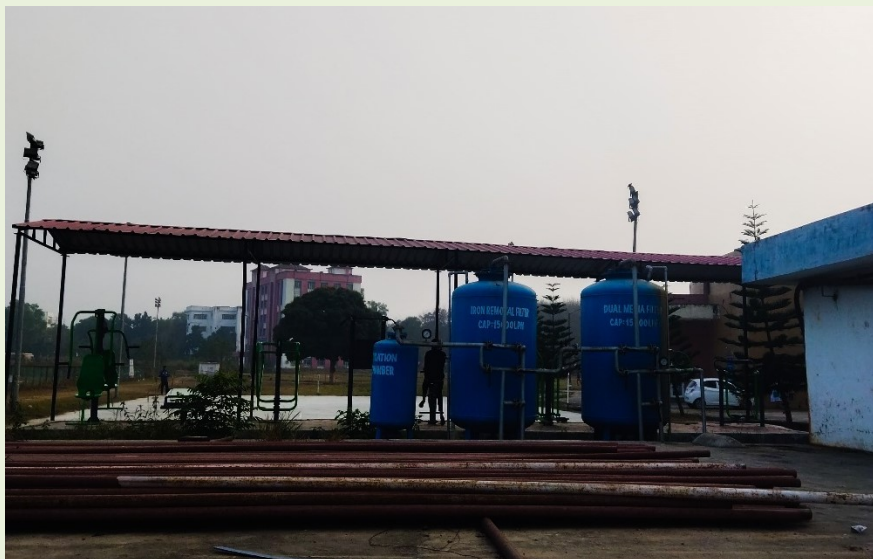
Figure 6: Iron Removal Filter unit
