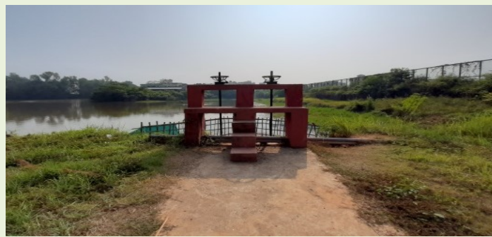
Fig. 6: Sluice gate for sustaining and controlling flow/water level of the TU Lake
