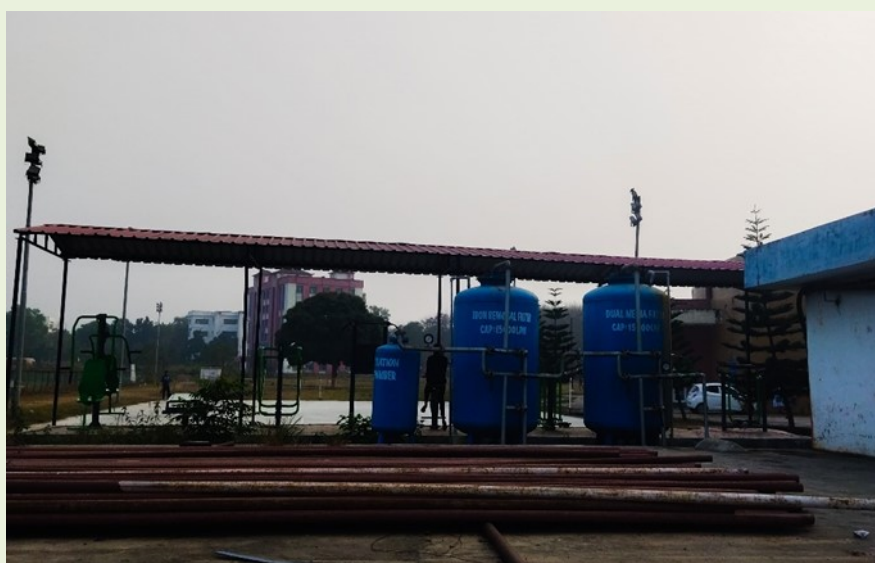
Fig. 4: Water treatment facility
