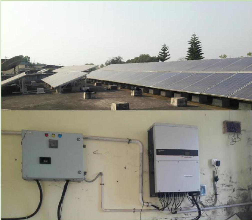
Fig. Use of solar power panels in TU Campus
