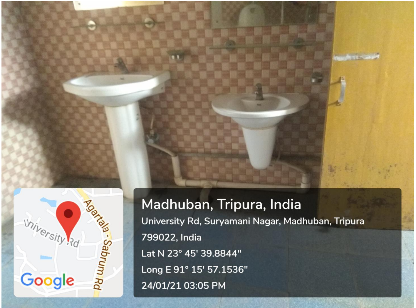
Disabled friendly washroom
