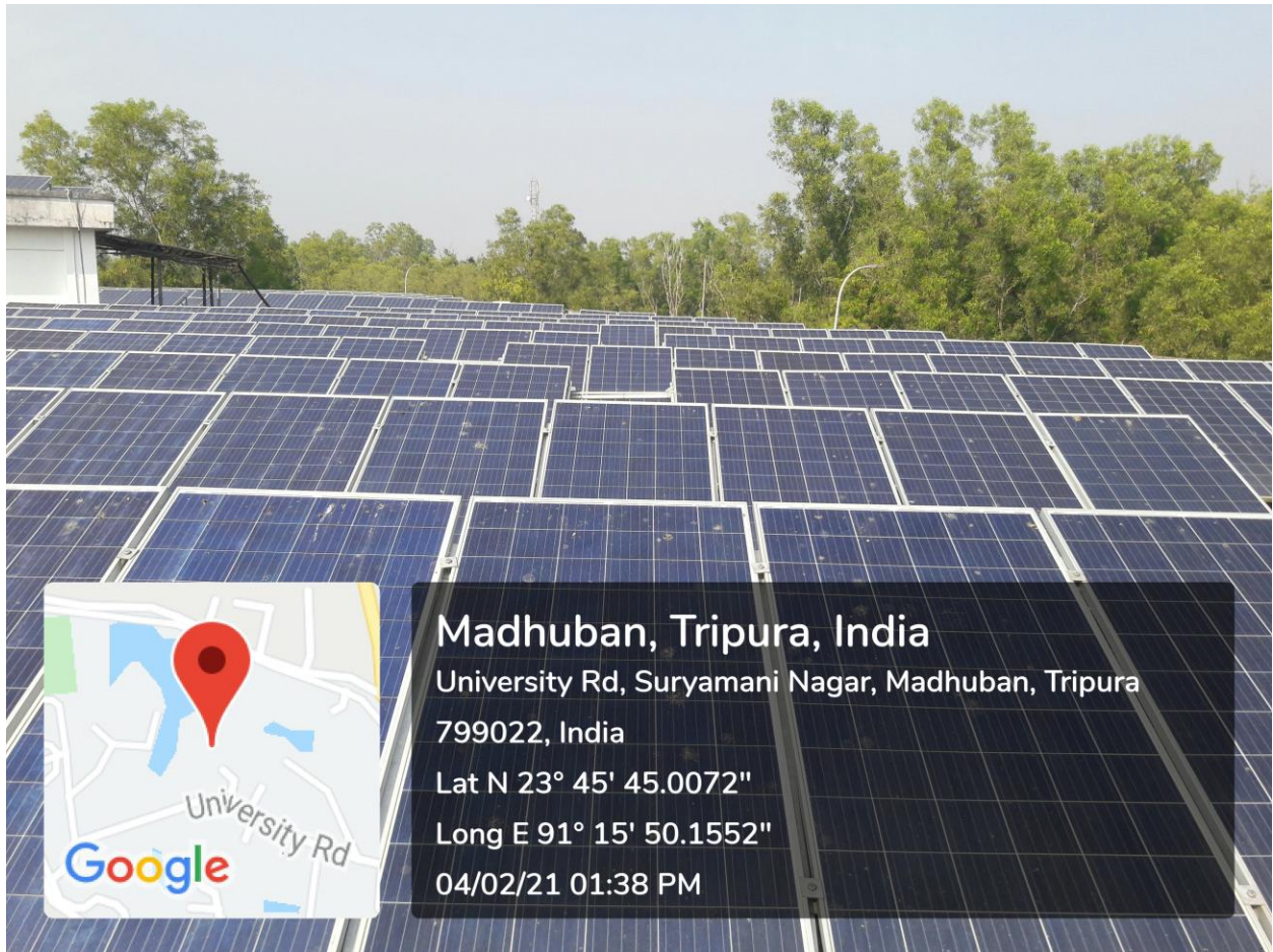
Solar plate installed in the roof top of each building
