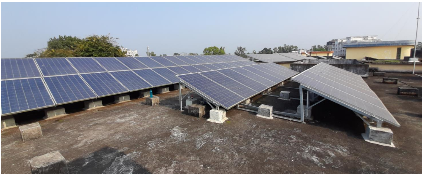
Solar plate installed in the roof top of each building
