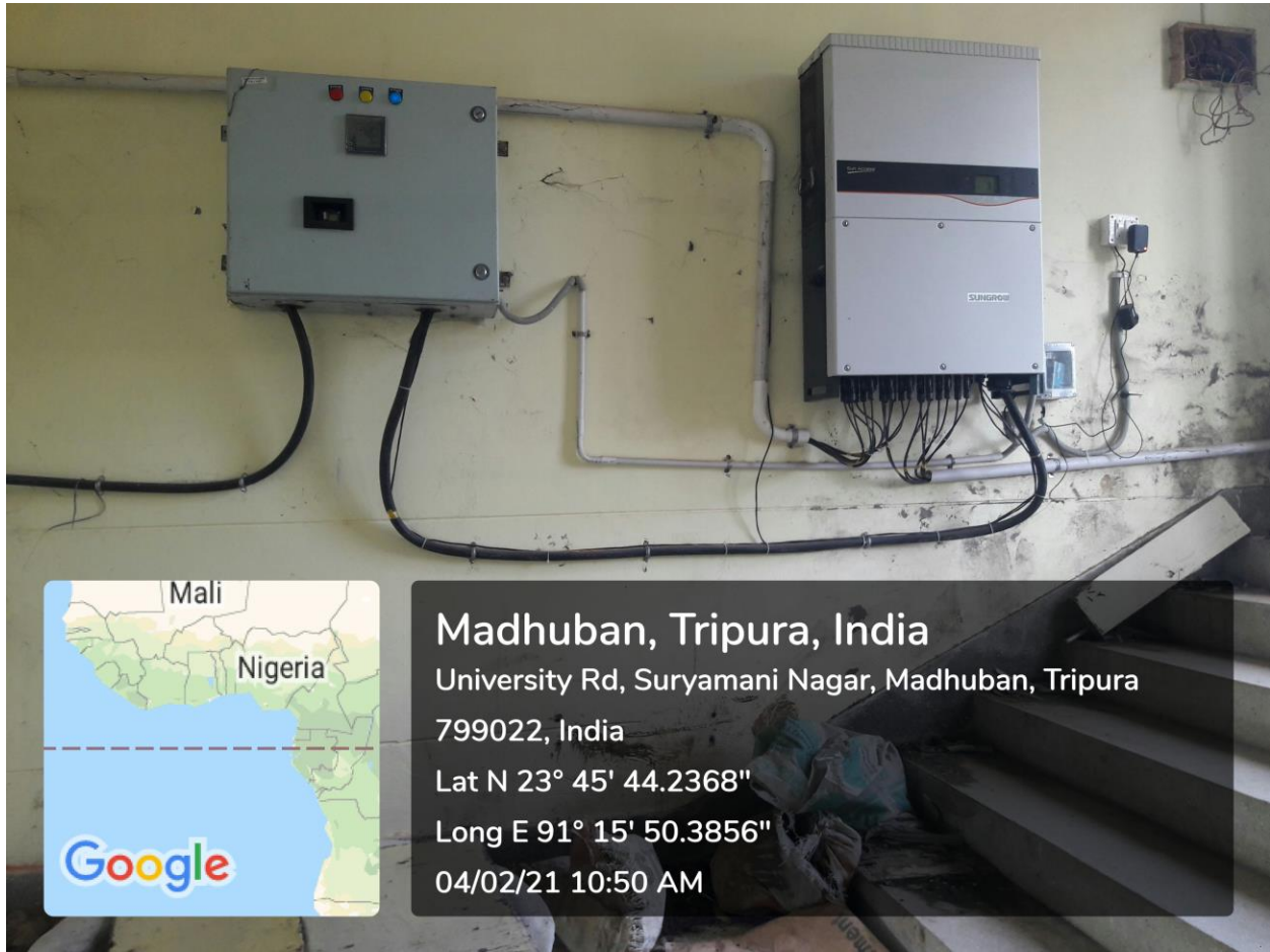
Solar plate installed in the roof top of each building connected to single box
