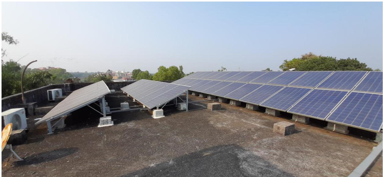
Solar plate installed in the roof top of each building
