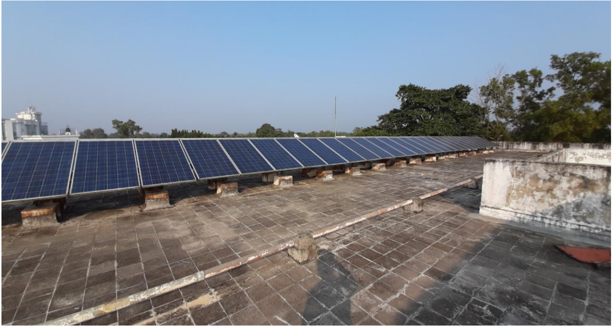
Solar plate installed in the roof top of each building
